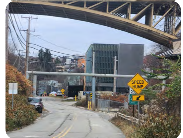
Overhead steam line
