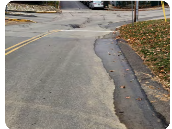
Stormwater pooling near intersection
